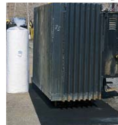
Ideal underneath leaking transformers.
